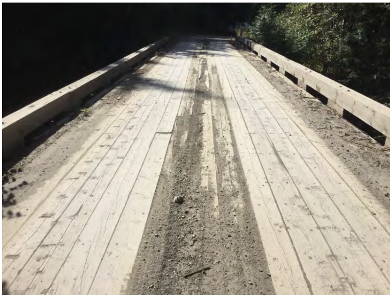
Middle 3 and outside 2 rows of planks were not replaced
